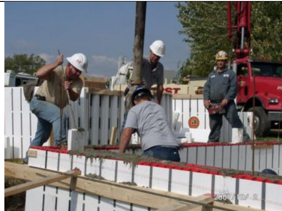
Figure 15 Pouring the ICF walls. 2 inches polyurethane insulation was sprayed over outside of ICF walls
