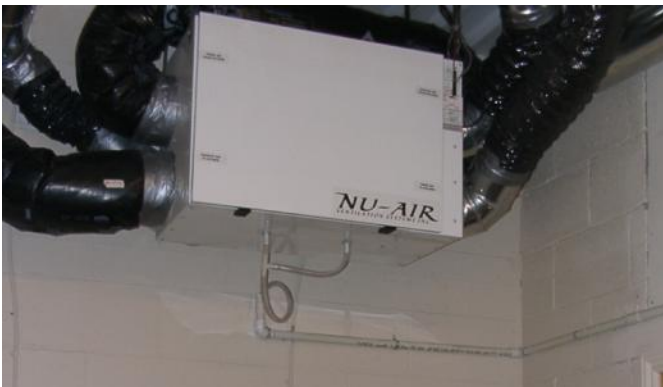
Figure 12 Heat Recovery Ventilator in workshop
