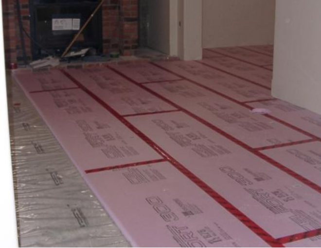
Figure 13 1.5 inch rigid foam board was used under the hardwood flooring, concrete pavers and slate tile bathrooms.
