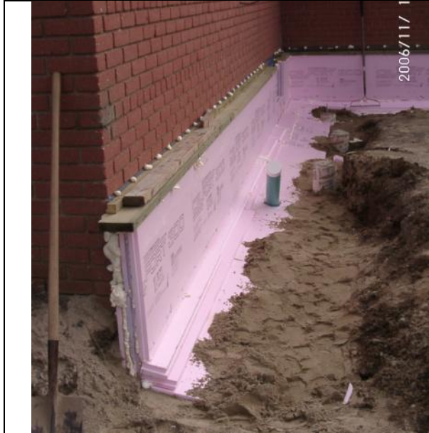
Figure 23 insulation reduces slab heat loss. Note how Larsen Truss will cover the edge of slab insulation
