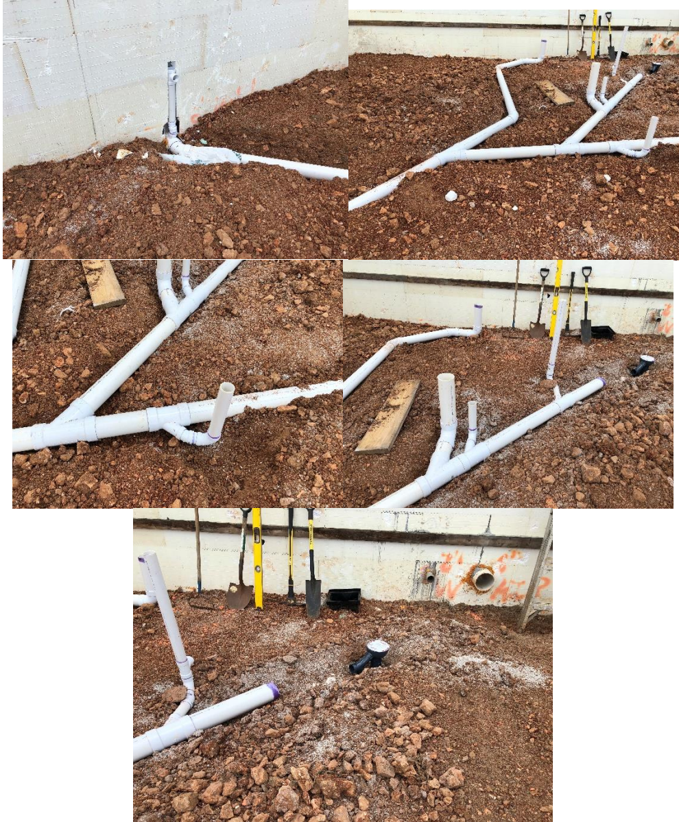
Pretty standard plumbing, nothing remarkable here really. In the rear of the last photo there is a 6" make-up air tube for fresh air, and a wall penetration for the potable water intake. Excess cooling water will also exit here and into the drain tile system which when collected in a cistern will be used to water the yard and the garden.
